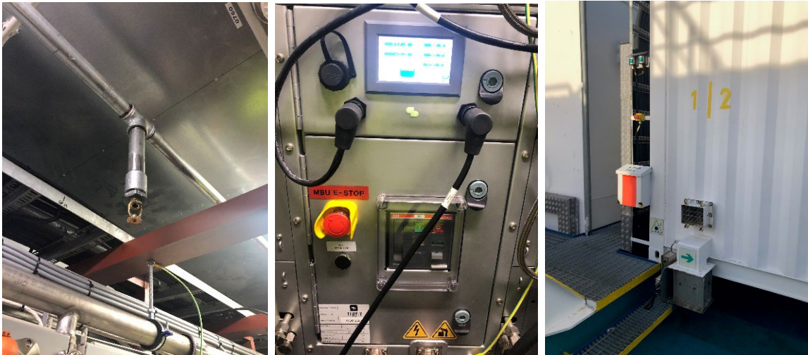
Figure 7 Sprinkler inside the battery container (left); emergency stop on a battery rack (middle); emergency stop outside battery container (right).
