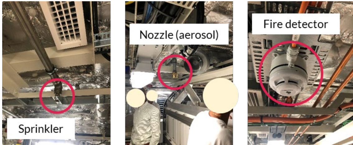
Figure 9 Safety systems located inside the battery room.
