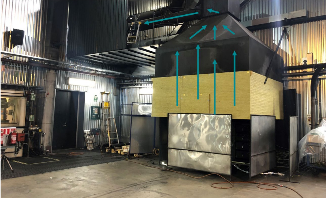
Figure 17 Standardised rack underneath the exhaust hood. The arrows indicate the movement of gas extraction
