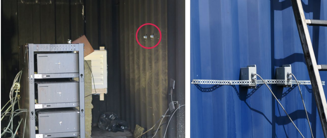
Figure 41 Sensing elements for the gas alarms (encircled) were inside the container while the alarms were on the outside
